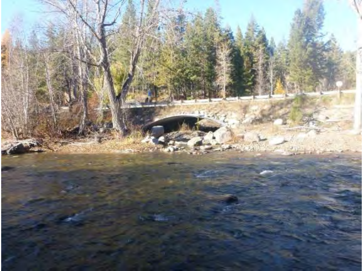
Figure 31 Sediment accumulation in the bottomless culvert at the confluence of the Little Bridge Creek tributary and the Twisp River.
