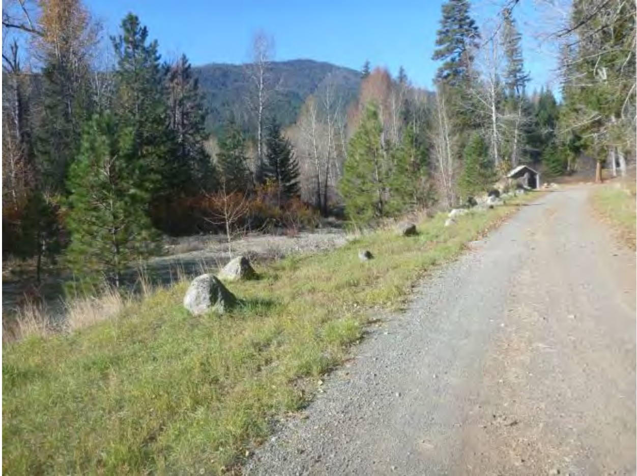
Figure 94. Gravel road and clearing and grading along river left corresponding to RM 17.8 to 18.0
